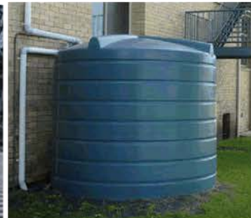
Rain Water Tank/s
